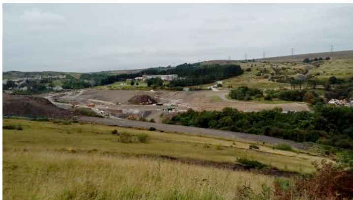
Figure 1: The former Control Data Corporation Site in Brynmawr, Gwent, during construction of the Heads of the Valley Road, summer 2016. Photograph by Kerry Pendergast.
