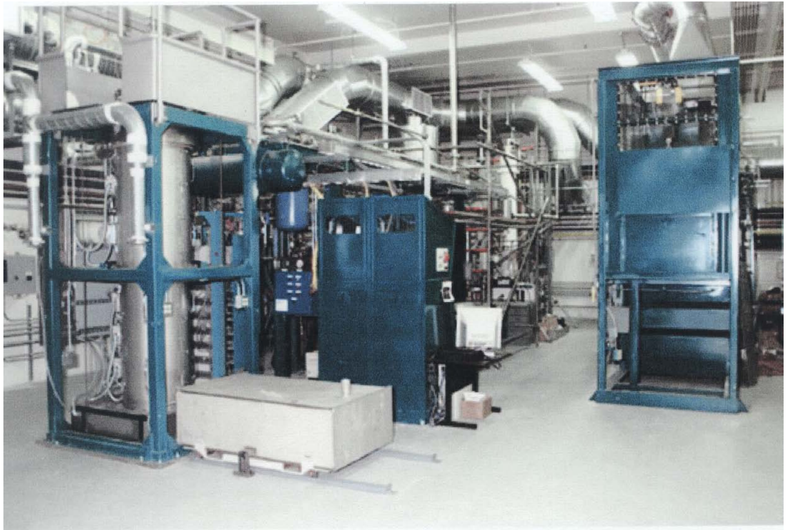
Integrated MSO system showing reaction vessel, off-gas treatment system, salt recycle system, feed preparation equipment and ceramic final waste forms immobilization system
