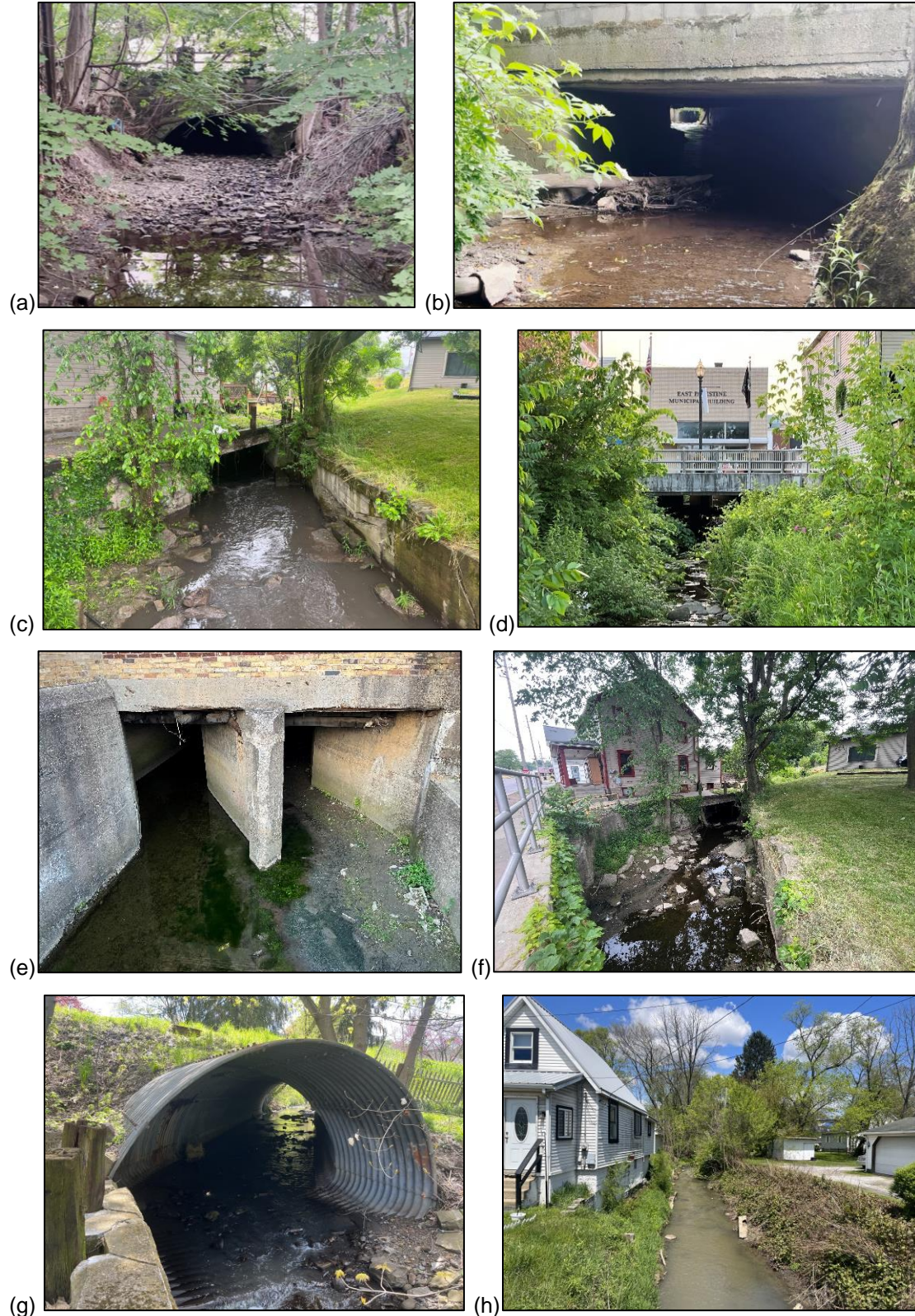
Figure ESI-17. Concrete and metal culverts transport Sulphur Run water underneath and adjacent to East Palestine roadways, properties, as well as commercial, residential, and municipal buildings.
